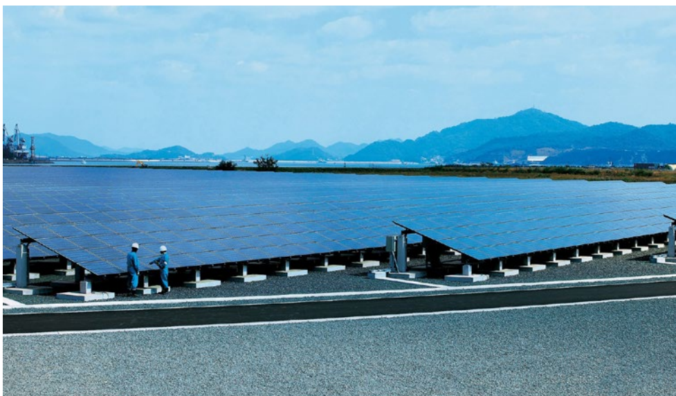
Fukuyama Solar Power Station (Chugoku Electric Power Co.)
