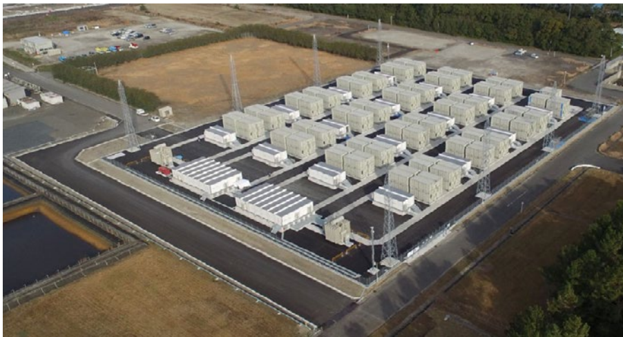
Buzen Battery Electrical Substation (Kyushu Electric Power Co.) Output: 50MW, Capacity: 300MW (operation started in March 2016)
