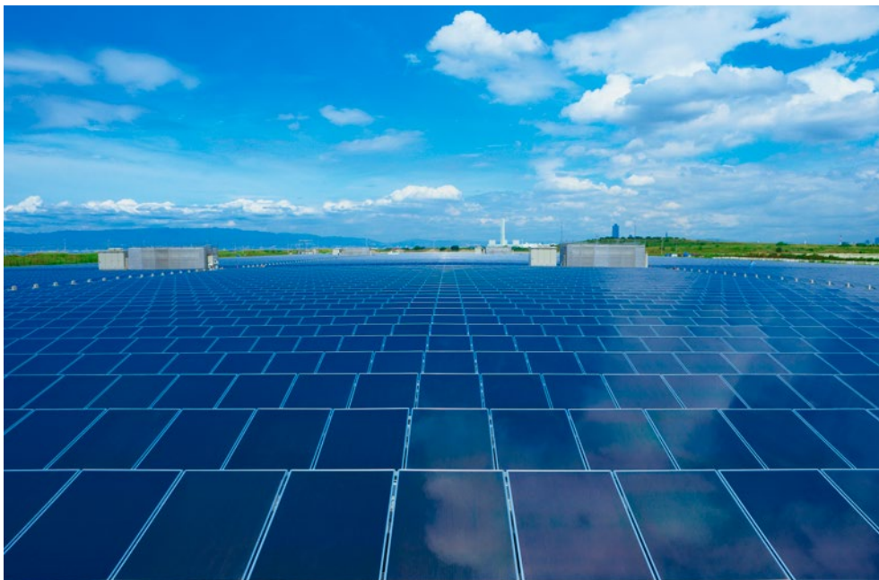
Sakai Solar Power Station (Kansai Electric Power Co.)
