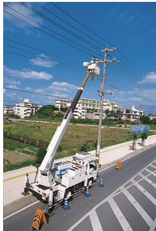
Power distribution equipment (Okinawa Electric Power Co.) Maintenance work in preparation for a typhoon
