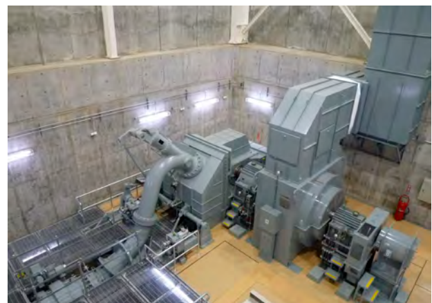
Katakai Betsumata Hydro Power Station (Hokuriku EPCo)
