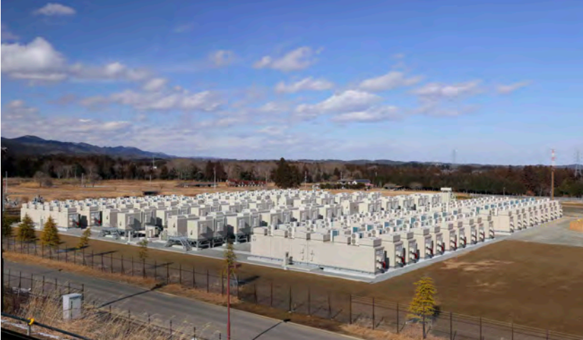
Storage battery pilot plant at Minamisoma Substation (Tohoku EPCO)
