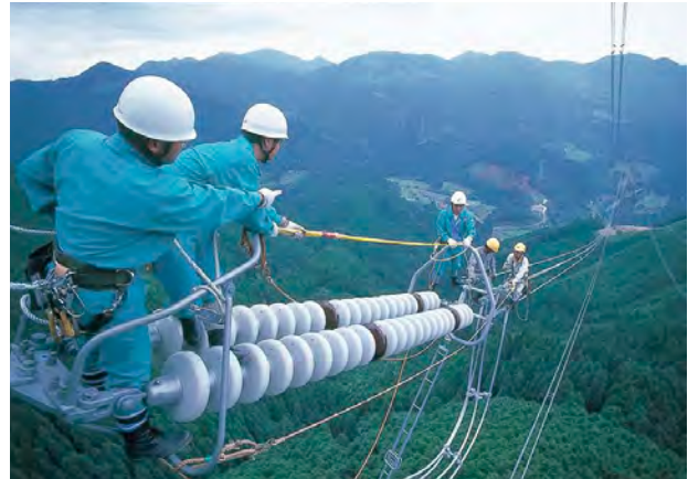
Maintenance of transmission systems (Chugoku EPCo)
