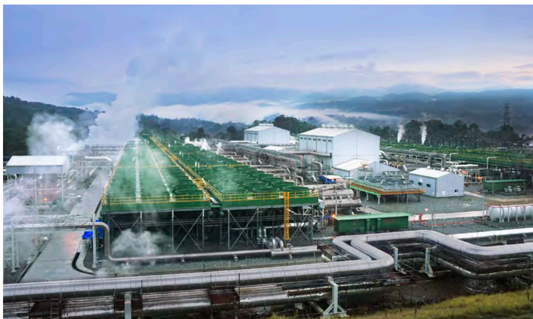
Sarulla Geothermal Power Plant (Sarulla Operations Ltd., a joint venture of Kyushu EPCo, ITOCHU Corporation, INPEX CORPORATION, PT Medco Power Indonesia and Ormat Technologies, Inc.)
