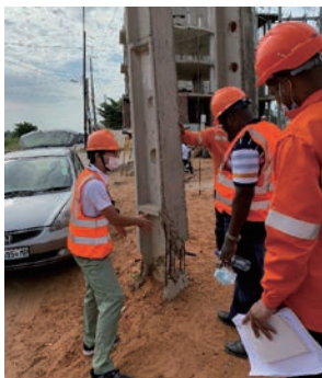
Technical Transfer on EDM's power distribution sites
