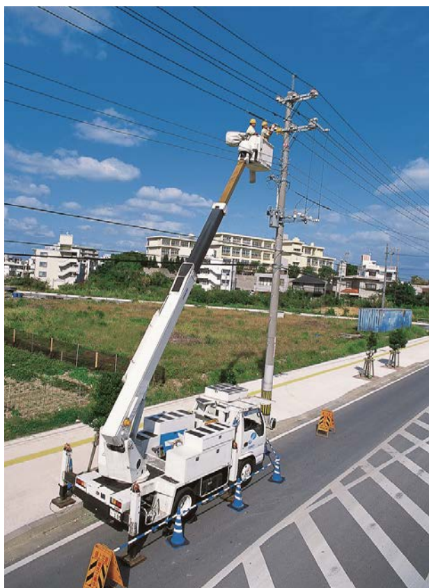
Power distribution equipment (Okinawa Electric Power Co.) Maintenance work in preparation for a typhoon
