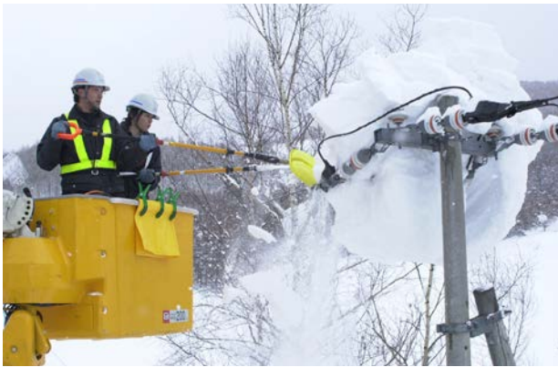
Removing snow from power lines (Hokkaido Electric Power Network)
