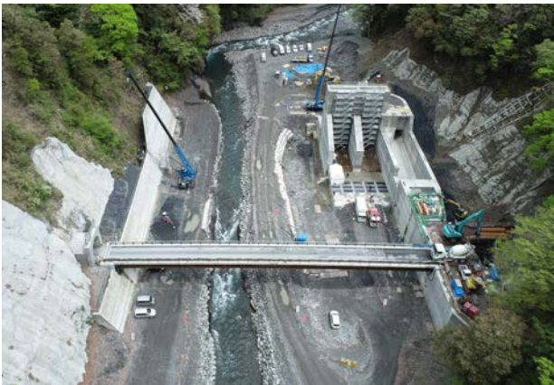
Abekawa Hydroelectric Power Station (Chubu Electric Power Co.) Official name: Abekawa Hydroelectric Power Station / COD: December 2024 (scheduled) / Owner: Chubu Electric Power Company
