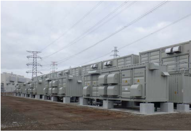
A large-scale storage battery (a redox flow battery) (Hokkaido Electric Power Network Co.,Ltd.) COD: April 1,2022 / Owner: Hokkaido Electric Power Network Co.,Ltd. / Site: Minami-Hayakita Substation, Hokkaido Electric Power Network / Power: 17,000 kW; Capacity: 51,000 kWh
