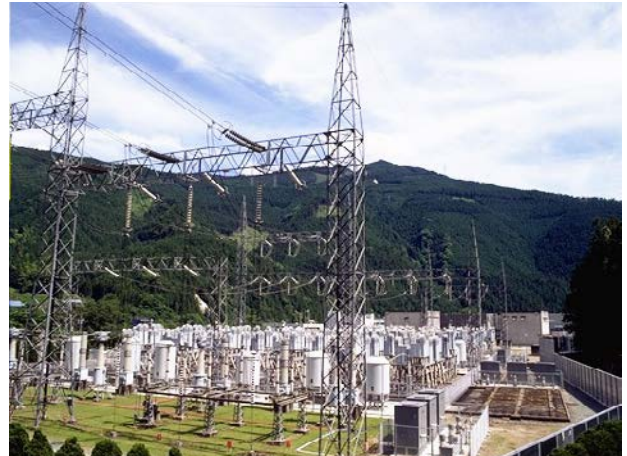
Sakuma Frequency Converter Station (Electric Power Development Co., Ltd. (J-POWER)) COD: 1965 / Owner: J-POWER Transmission Network Co.,Ltd. / Transmission Network / Capacity: 300MW
