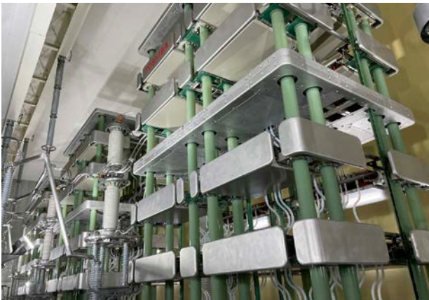
Thyristor Valve in the New East-West HVDC interconnection at the Shin-Shinano substation (2021) (Tokyo Electric Power Company Holdings, Inc.)
