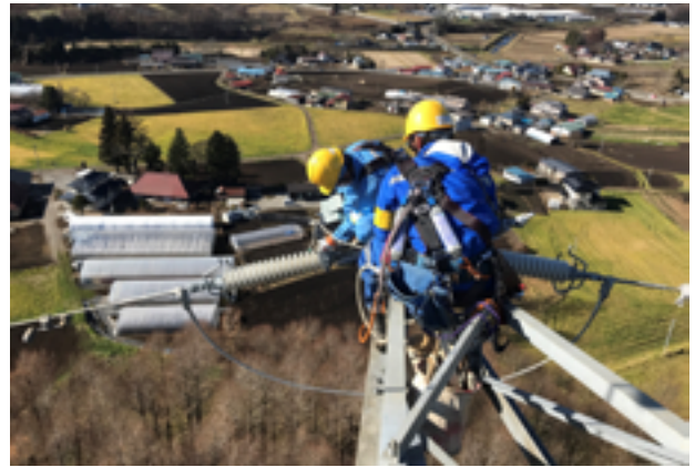
Power transmission line maintenance (Tohoku Electric Power Network) Maintenance of transmission and distribution equipment for stable power supply
