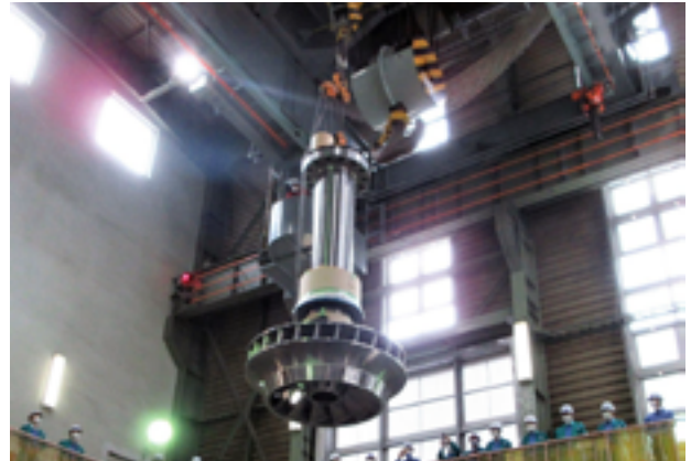
Hydro turbine runner suspended for repowering (Chugoku Electric Power Co.) Site: Takiyamagawa Power Station / COD: January 1959 / Output: 52.5 MW
