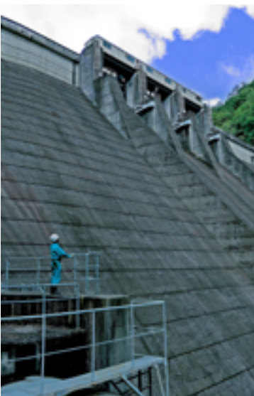
Available storage capacity doubled by heightening dam (Chugoku Electric Power Co.) Site: Odomari Dam / Completion: July 1935 / Height increase: April 1959
