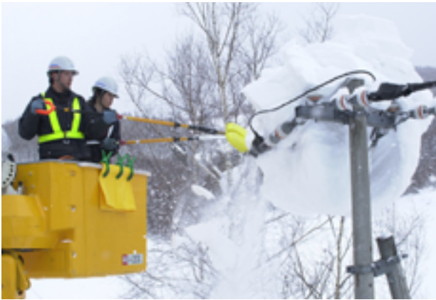
Removing snow from power distribution lines (Hokkaido Electric Power Network)
