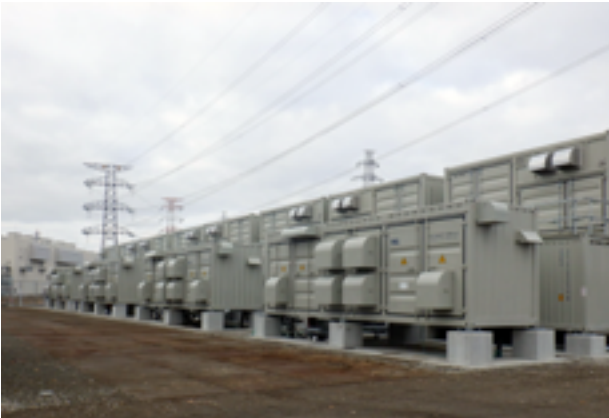
A large-scale storage battery (a redox flow battery) (Hokkaido Electric Power Network Co., Ltd.) COD: April 1, 2022 / Owner: Hokkaido Electric Power Network Co., Ltd. / Site: Minami-Hayakita Substation, Hokkaido Electric Power Network / Power: 17,000 kW; Capacity: 51,000 kWh
